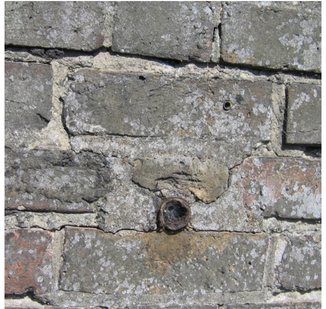
Look closely to spot the pipes of the flame defile device © John Guy
